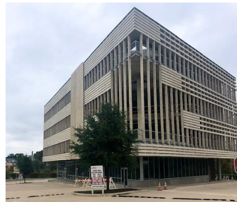
BookMark Center retail and office space under construction as part of Half Price Books' multi-phased development
