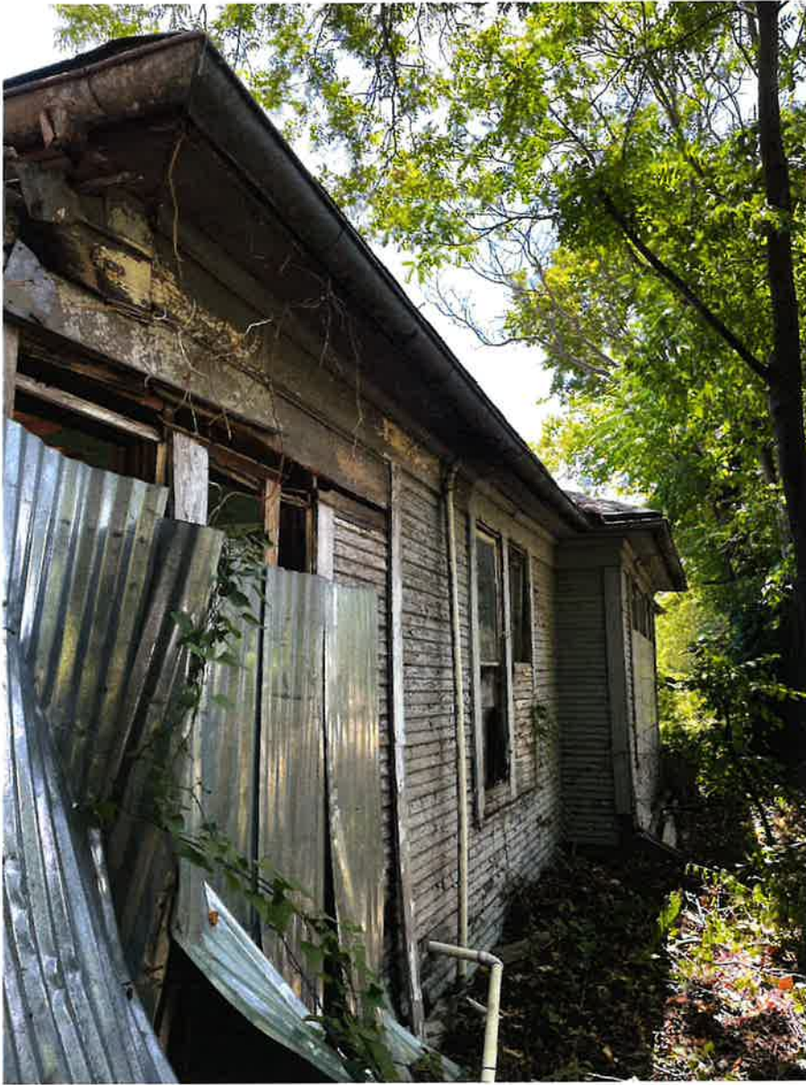
Figure 21 - Partial view of the north side of the subject property (photograph taken July 25, 2022)
