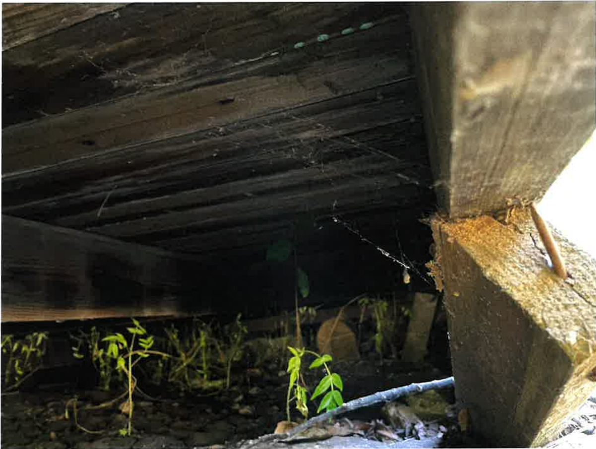
Figure 9 – View gained from one of several areas showing the underside of the structure (photograph taken July 25, 2022)
