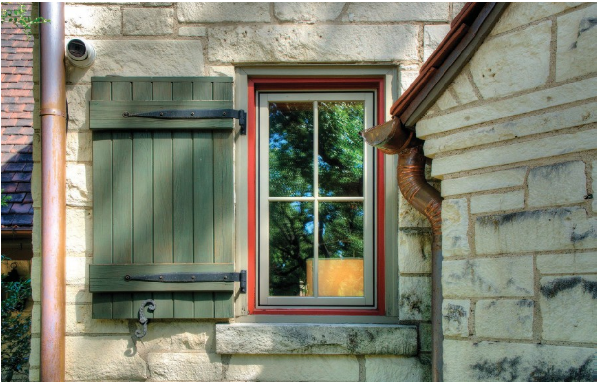
Figure 13: Detail of non-historic window and historic shutter on south façade. July 2021. Photography by Carolyn Brown.
