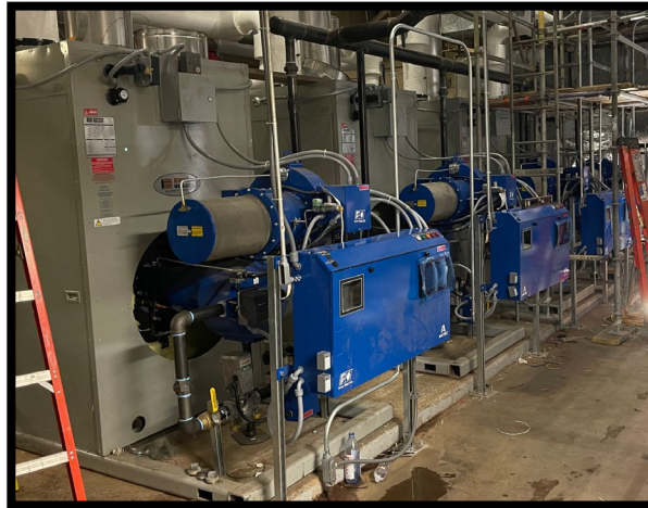
Dallas City Hall Hot Water Boilers (New)
