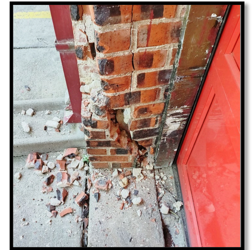
Fire Station #45 Structural damage
