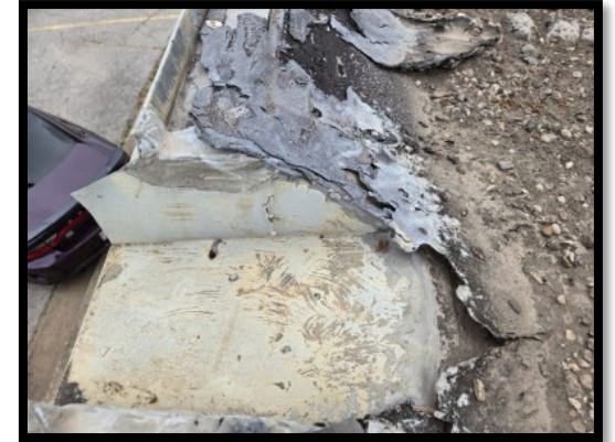
NW Transfer Station Roof Deteriorated flashing
