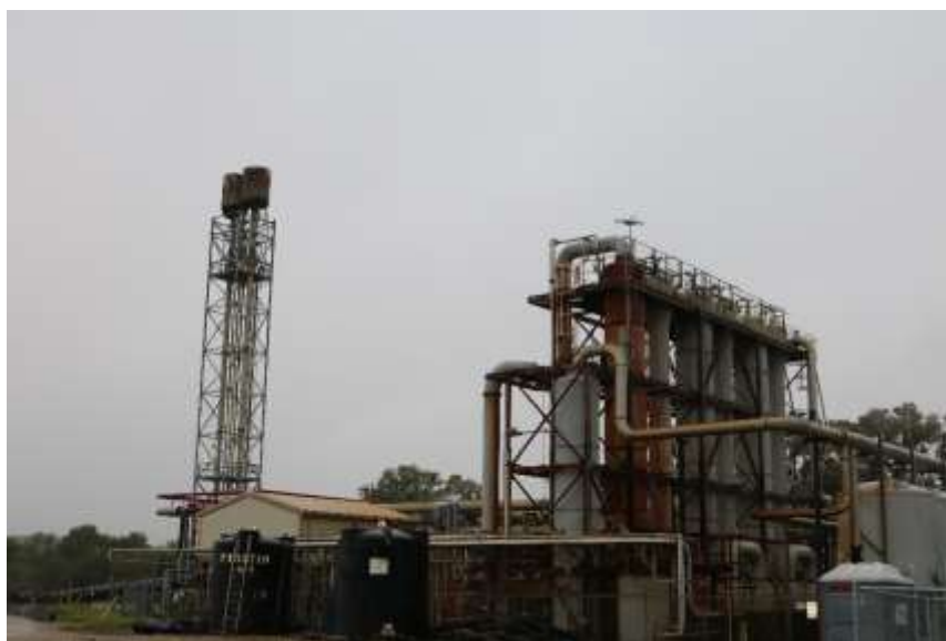
Figure E-19: Landfill Gas-to-Energy Plant
