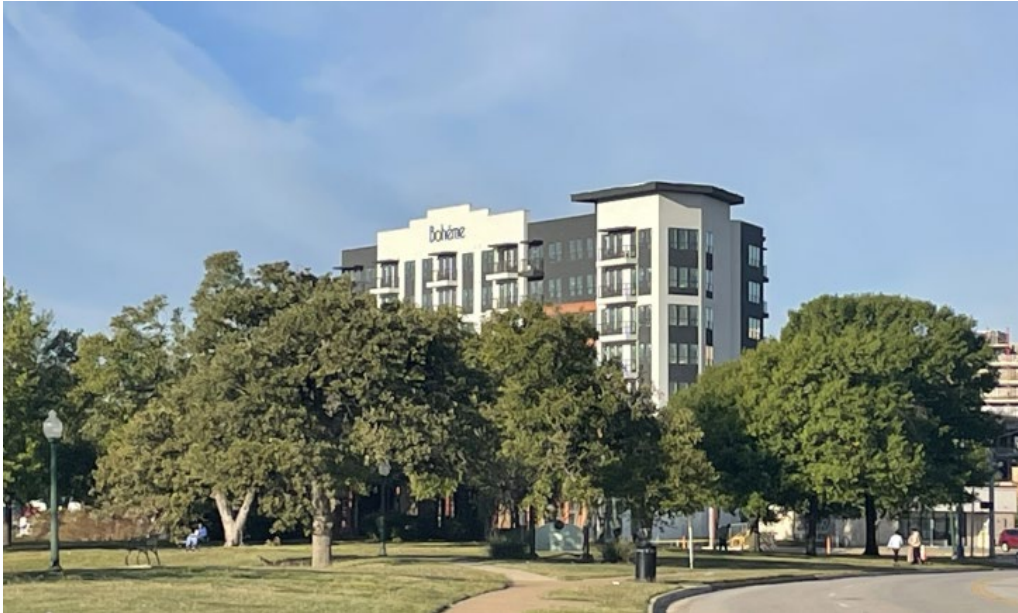
View from Lake Cliff Park looking toward the Boheme Apartments under construction at 1207 N. Zang Boulevard (formerly the site of El Fenix Restaurant).
