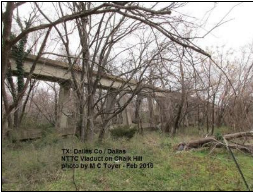
Figure 5. Photo showing the bridge substructure (courtesy of M C Toyer, February 2016, https://bridgehunter.com/tx/dallas/bh67825/ ).
