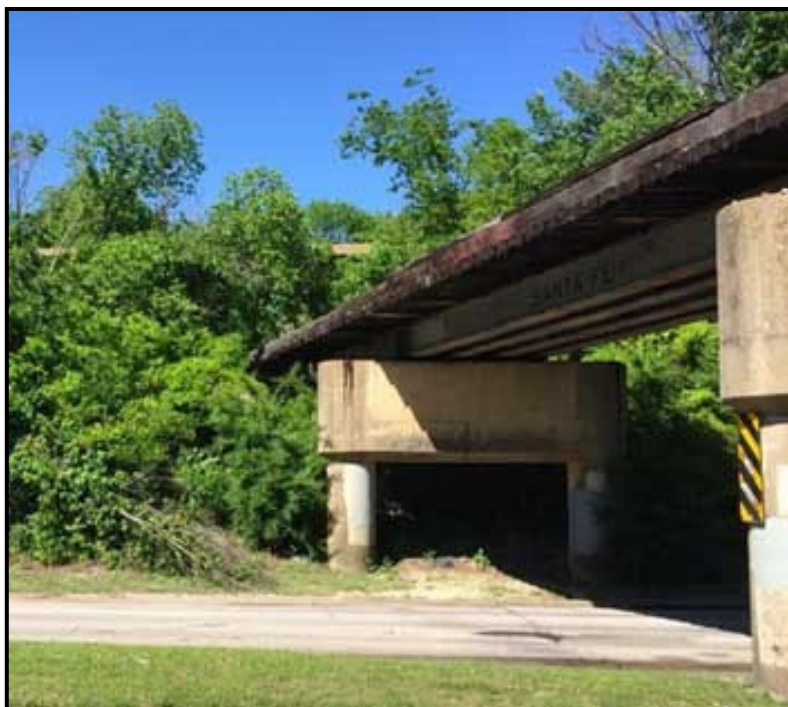
Figure 12. The triple overpass from Jefferson Boulevard at grade, under the Santa Fe railroad bridge with the Mountain Creek interurban bridge in the background (photo taken April 25, 2015).
