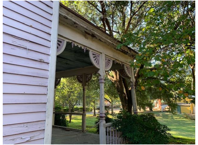
North Elevation – Failing soffits and Decorative elements
