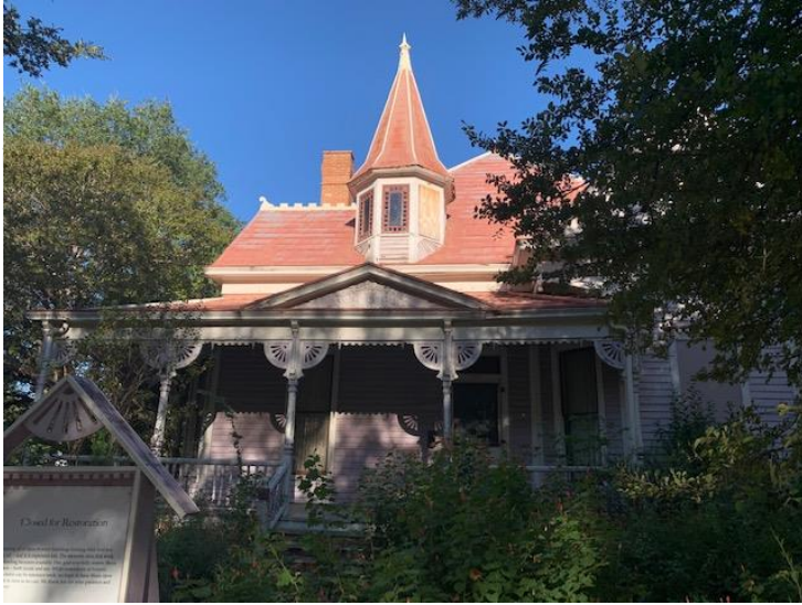
South Elevation – Roof wear visible
