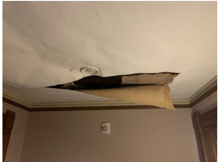
Interior – Ceiling Failure
