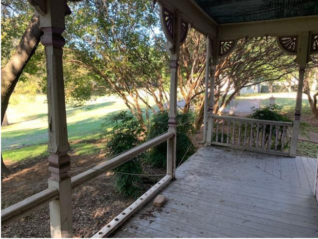
West Elevation – Failed Porch
