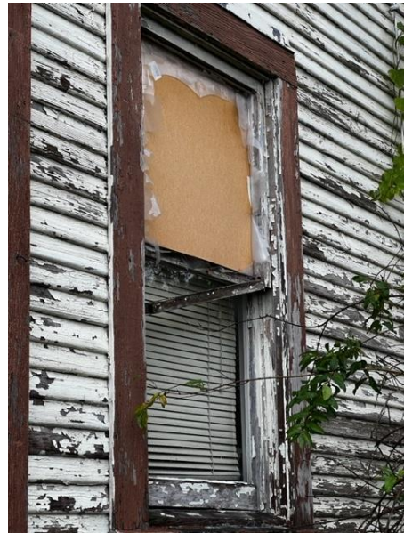
North Elevation – Failed Window
