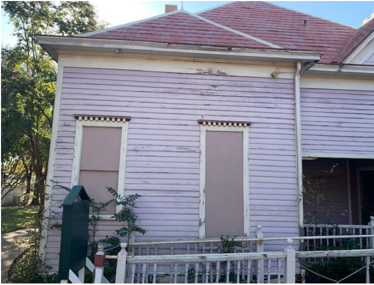
North Elevation – Failed Windows and ADA ramp
