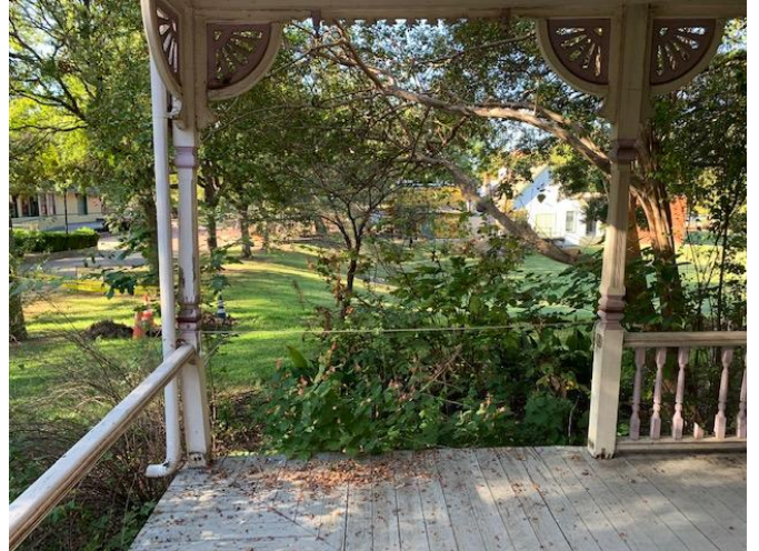
West Elevation – Failed Porch
