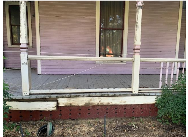
West Elevation - Failed porch section
