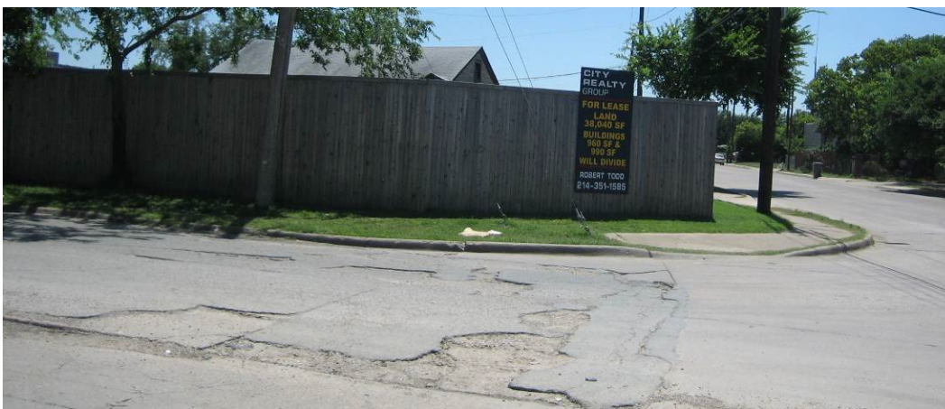
Crumbling streets and non-contiguous sidewalks
