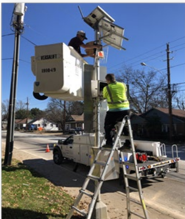
Breathe Easy Air Quality monitor installation at Exline Recreation Center
