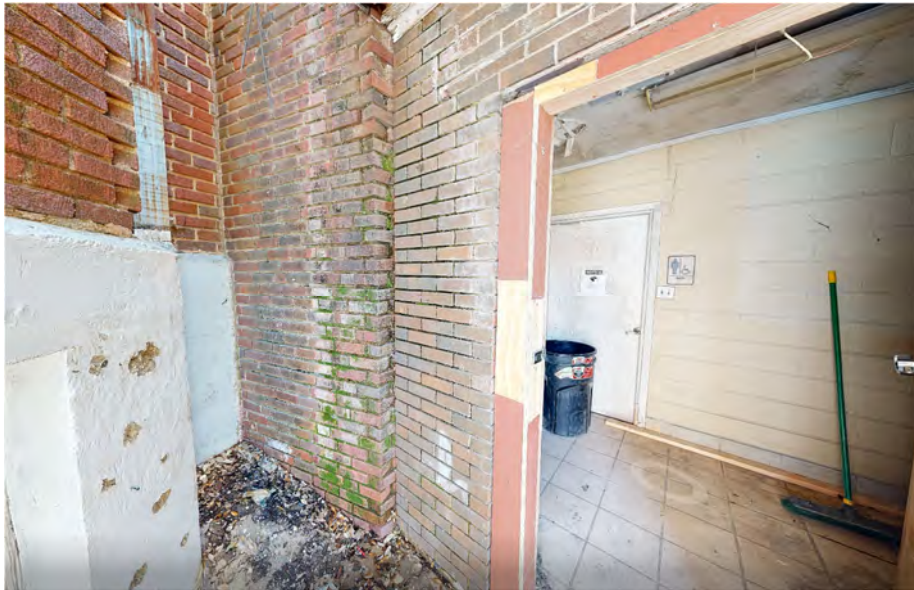
Figure 5 Entrance Addition on the right and Sanctuary on the left. Note the construction joint between structures, different brick material, and misalignment of mortar joints.
