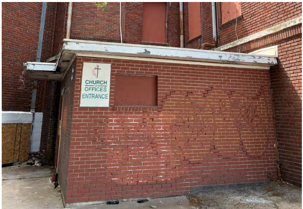
Figure 3 Overall view of Entrance Addition. Note the poor quality of construction including plywood roof and soffit.
