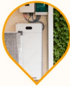
Solar Energy Storage
