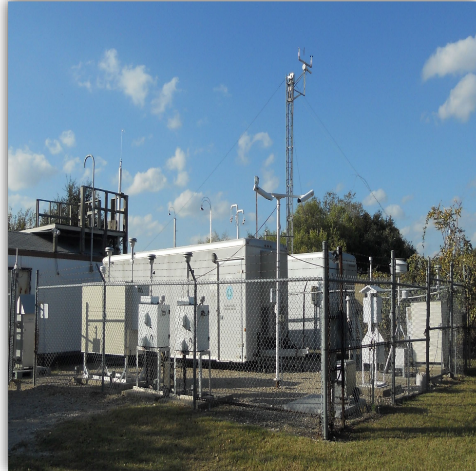
Dallas Hinton Air Monitoring Site
